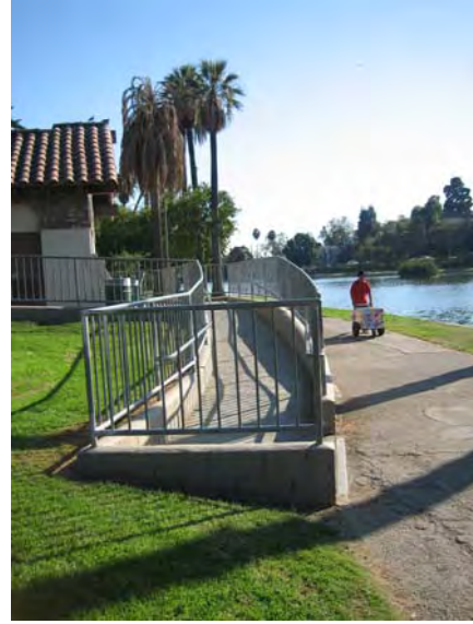
Plate 39. Ramps near Boathouse Restrooms
